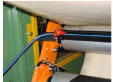
The anti-static bar, showing an electrode and cabling.
